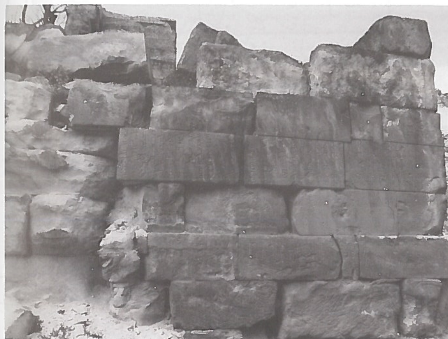
Fig. 6. The south wall of the vestry of the church of St Sergius at Ehnes (photo: A.N. Palmer, April 1990).
